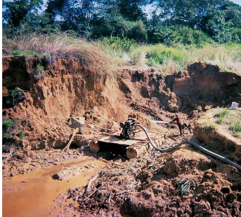
Figure 1. Water cannons are used to mine diamonds near the Quebrada River in the Guaniamo region of Venezuela. Photo by Ric Taylor.
